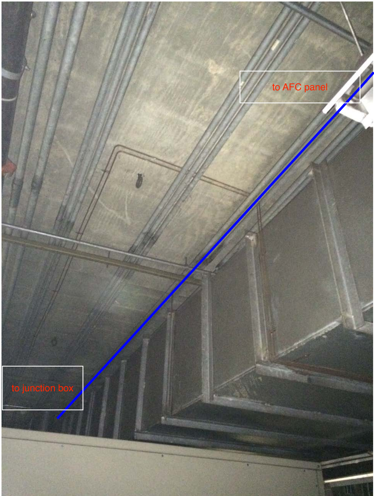
Photo #3 – G01 Benning Road: Conduit run from junction box inside AFC panel room
