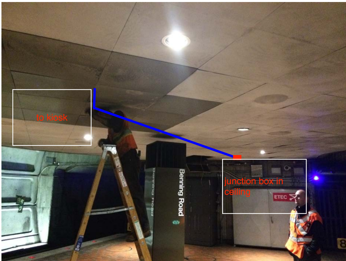
Photo #1 – G01 Benning Road: Ceiling tiles under kiosk where conduit run begins
